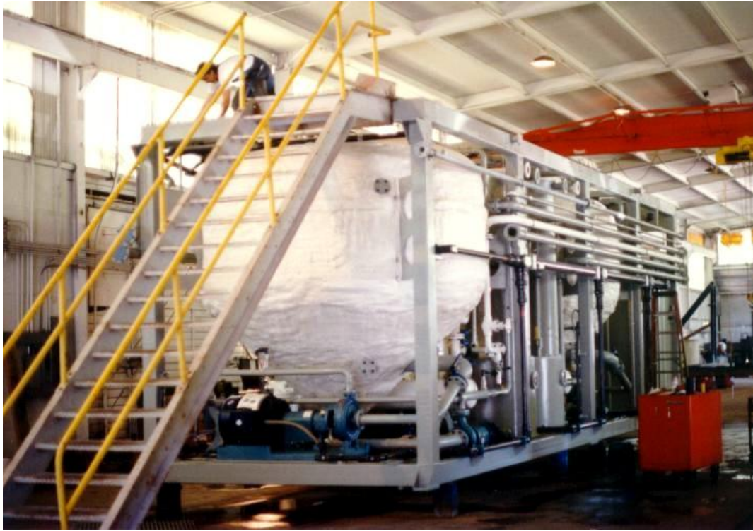
Photo 6. Washing system module installed in a wash shop
