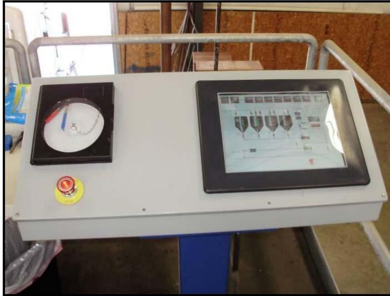
Photo 7. Control panel with touch screen
